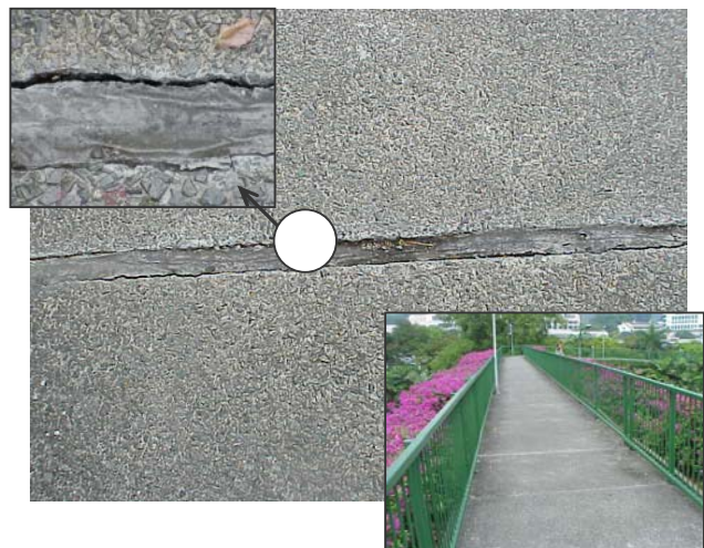
Figure 2. A length of failed commercial sealant on an overhead bridge.
